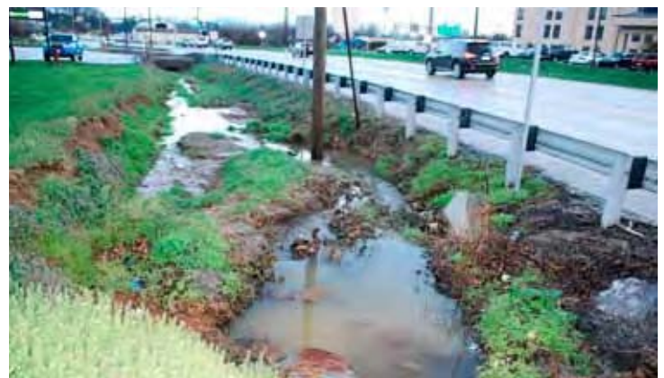
An enclosed surface water drainage facility under a township road in York County empties into a parallel open surface water drainage facility along a PennDOT highway. Trash and accumulated sediment lead to poor drainage in the upstream area. Photo by Michael H. Fleming, ISMF LLC.
