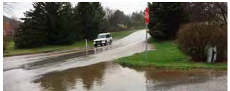
This open surface water drainage facility in York County is not functioning as designed due to paving overlay and inlet location. Photo by Michael H. Fleming, ISMF LLC.
