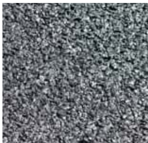
UTWC seals the pavement, reducing oxidation and weathering of the surface. It has a service life of 8 to 10 years. (PennDOT photo)
