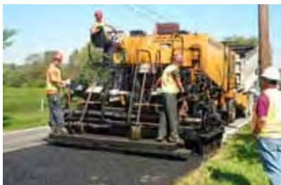
A single paving machine applies the polymer modified emulsified asphalt membrane overlaid with an ultra-thin bonded wearing course of hot-mix asphalt concrete in one pass. (PennDOT photo)
