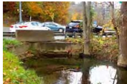
At an intersection of a state and township road in Allegheny County, PennDOT is planning to relocate a small bridge while improving an enclosed surface water drainage facility and headwalls. Photo by Harry Funk, The Almanac .
