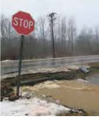
A subsurface water drainage facility in Warren County overflows after warm temperatures and heavy rainfall prove too great for the pipe under the road to handle. Photo by Stacey Gross, Times Observer.
